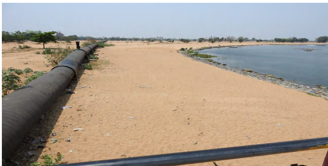
Figure 15: Water pipeline of IOCL standing on the dump as the supporting piles are buried under sand.
