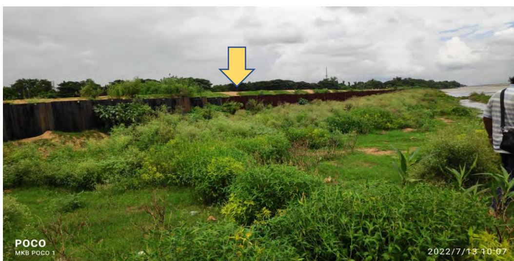
Figure 7: Dump (near Baliyatra ground) showing two levels of iron sheet piles - one pile at the higher level and other pile at lower level almost touching the shorelines.
